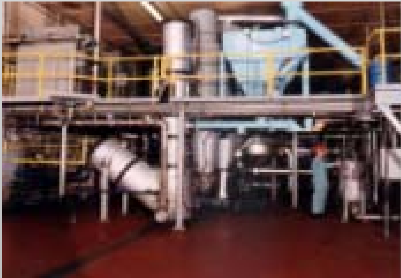
40 dry Tpd RTP
