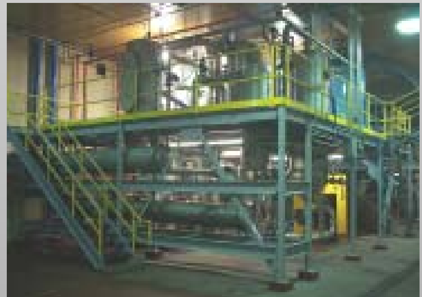
50 dry Tpd RTP
