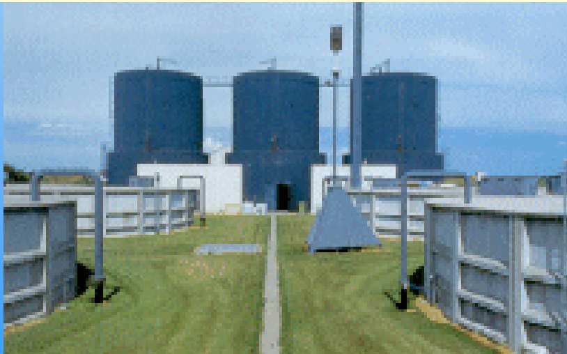
Lemvig centralised biogas plant, Denmark, producing about 4 million m 3 /year of gas Agores Website
