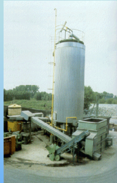
Dranco plant for anaerobic digestion of biowaste, Ghent, Belgium (supported under THERMIE) Agores Website
